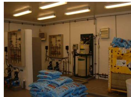
Grainger Springs Treatment Facility
